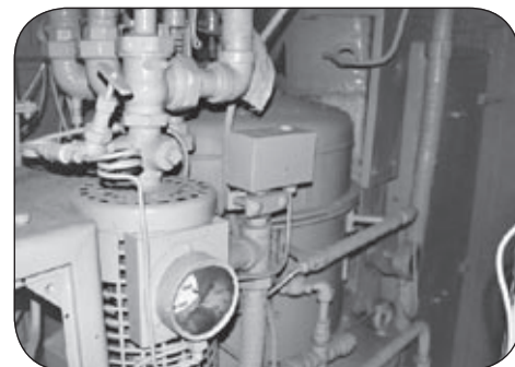
Steam generator on 4022/833.
